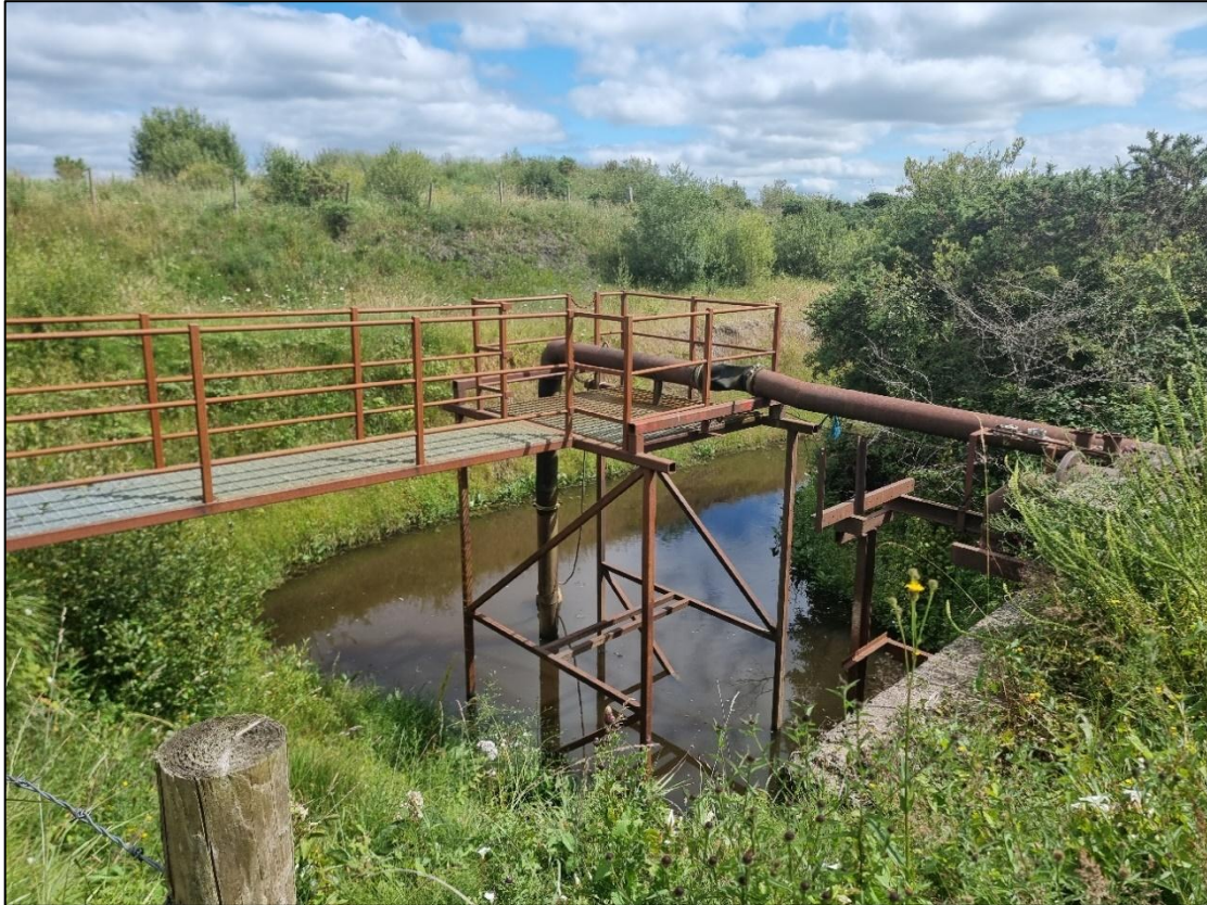
Plate 6-19 Pumping station and silt pond located in Ballydermot South Bog
